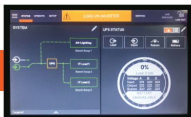
Shows real time feeder information such as voltage, current, harmonics, and power monitoring (kVA, kW, KVAR, & PF).
