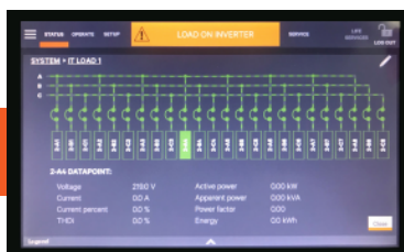
Power path status via animated single line mimic display shows the current status of main source breaker and distribution modules.
